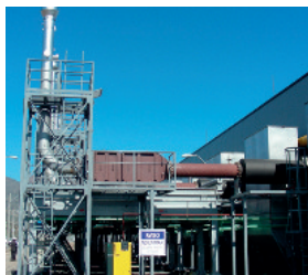
Emergency & Cogeneration Plants
