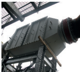
Waste Incineration Plants
